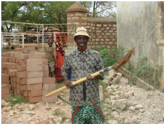
The construction of the new Outpatient Department at Bay Regional Hospital in Baidoa has been completed. The OPD will be run by IMC. Renovation of the Operating Theatre and X-ray room will start in August. Rehabilitation of Bay hospital is implemented by UNOPS with support from WHO.
