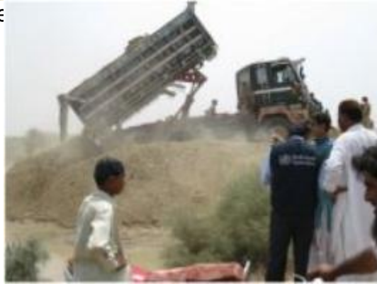
Work in progress to repair the road Thursday 25th of April 2024 04:01:15 PM
