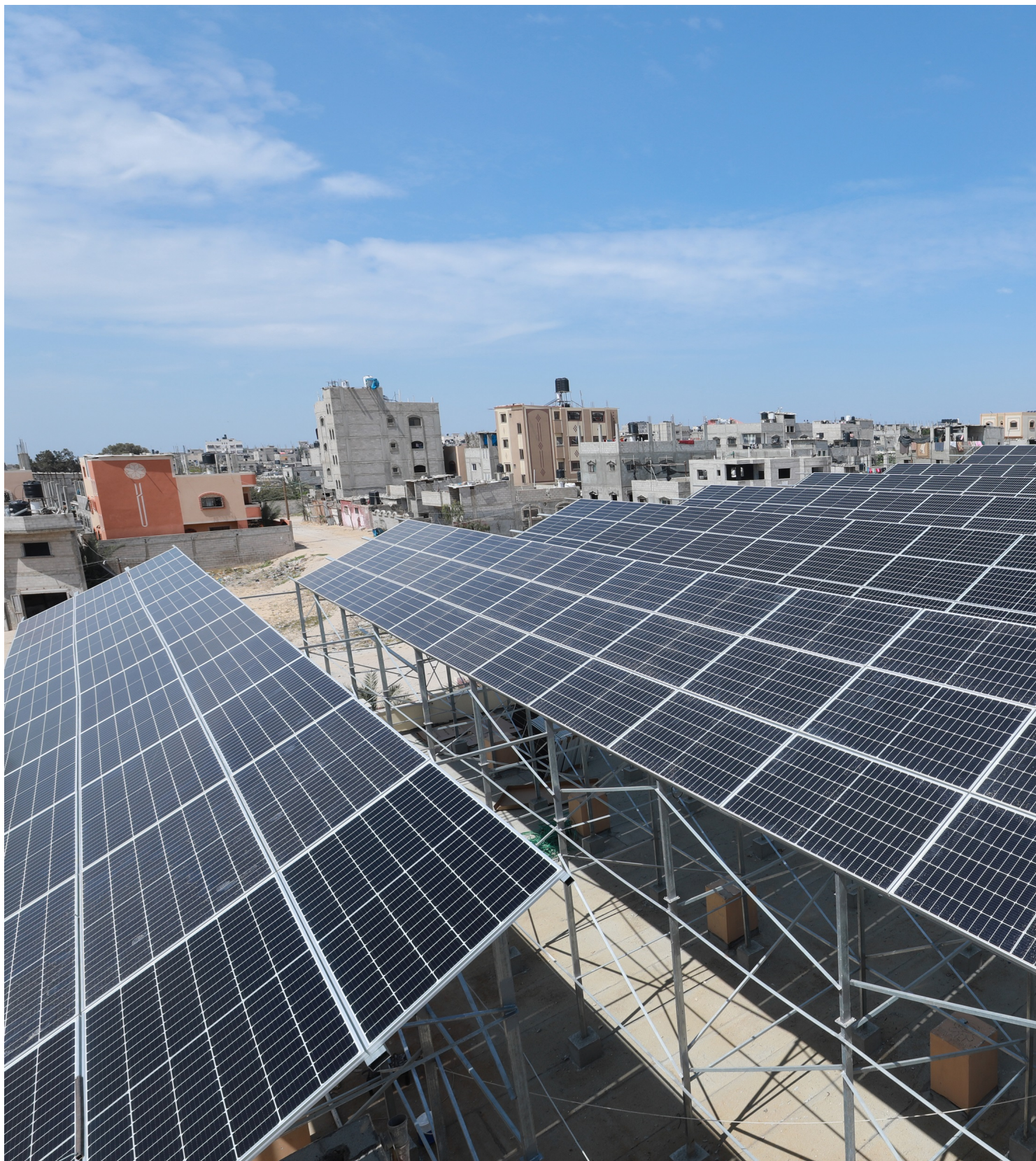
The solar power plant at Nasser Hospital in Gaza. Credit: WHO 17 June 2019, Gaza - The World Health Organization (WHO) and implementing partners inaugurated the newly installed
