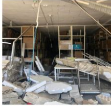
Heavily damaged central drug warehouse, WHO Lebanon
