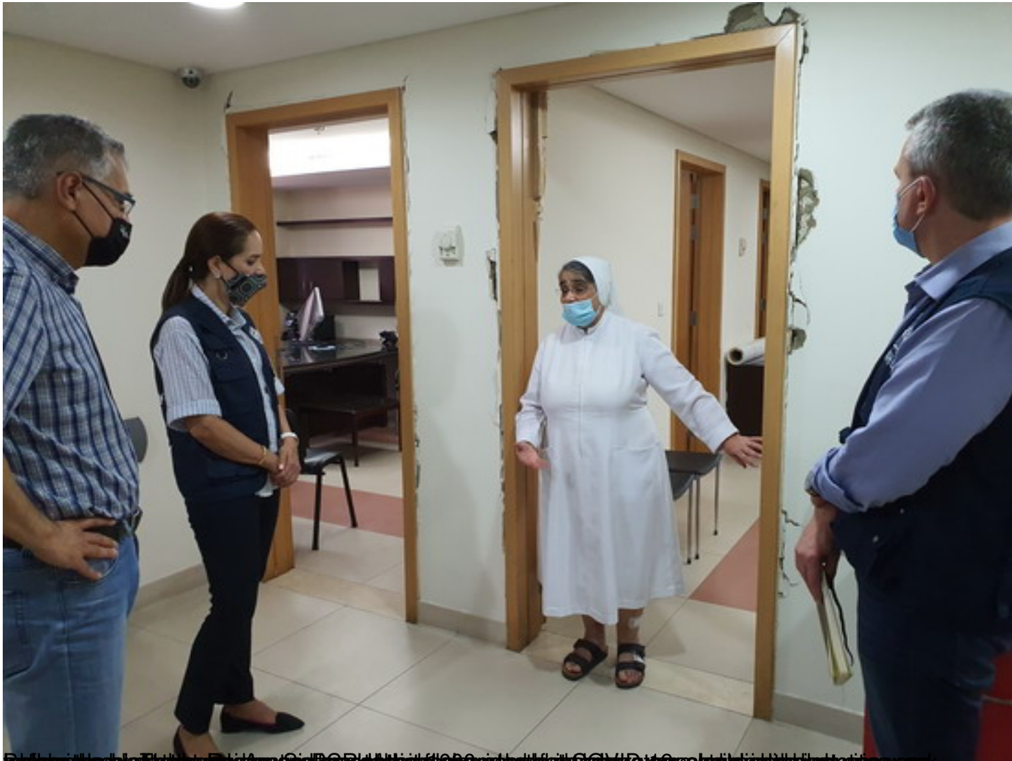
Dr. Hani El-Hayek, Director General of the Ministry of Health, visits the Rosary Sisters Hospital in Beirut, Lebanon, to assess the damage caused by the blast.
