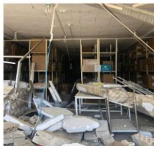
Heavily damaged central drug warehouse, WHO Lebanon
