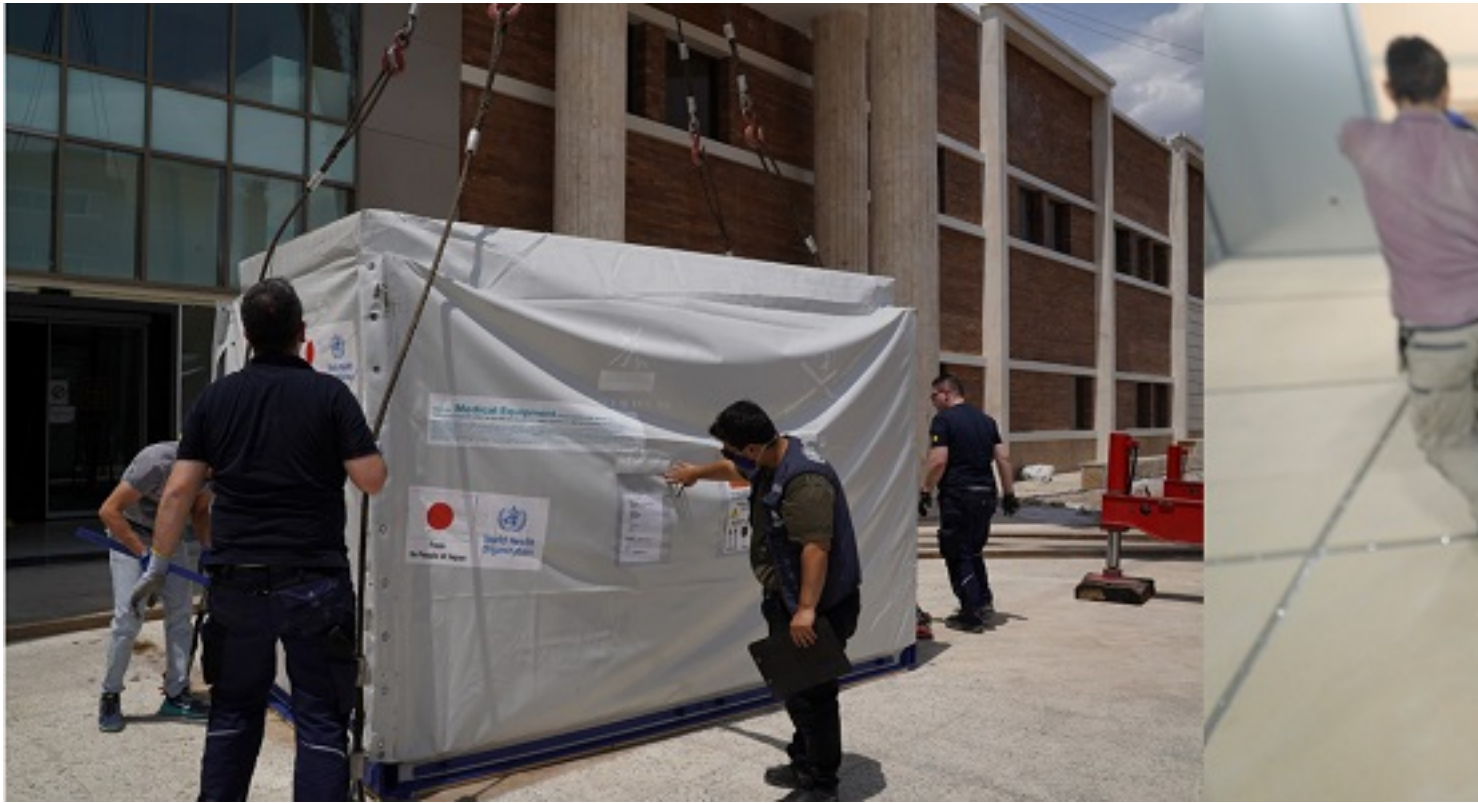
Unloading of the MRI machine and preparing for radio frequency shielding for MRI at Hajar Hospital in Shahrekord
