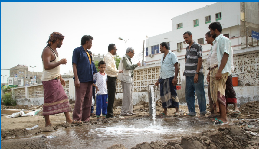
A water well has been drilled inside Al-Thawra Hospital with support of WHO to increase the water capacity of the hospital
