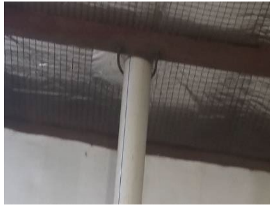
Protected ceiling at the treatment unit in Sa’adah (wool fiber glass insulation layer will be recommended for the steel roof)
