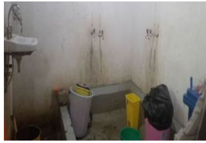
Drainage of the handwash basin is broken in Sa’adah
