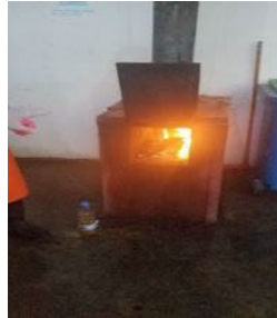
Safety box reducer chimney with un-protected fence in Sa'adah
