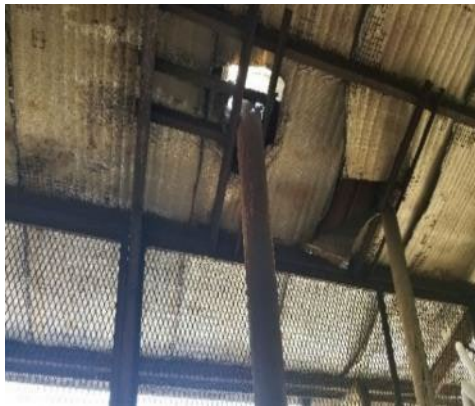
Burned ceiling with corroded and deteriorated chimney at the treatment unit in Hodeidah
