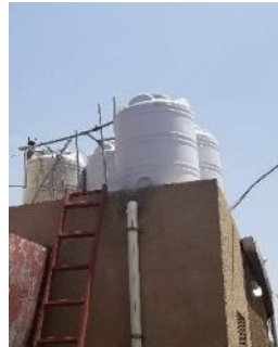
Roof plastic tanks in Sa’adah
