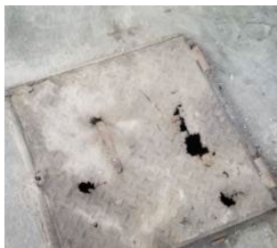
Corroded iron covers in Hodeidah
