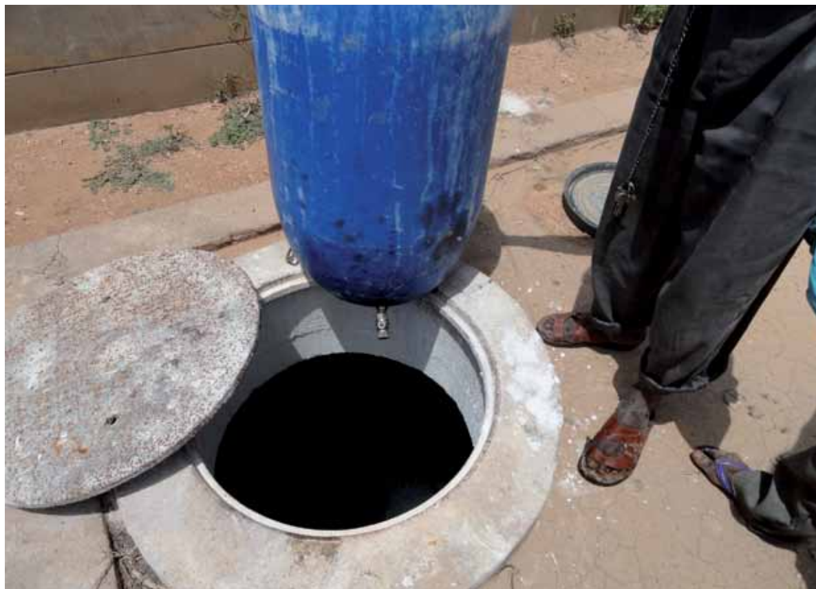
● Manual chlorination of water in a water facility, Hargeisa, Somaliland
