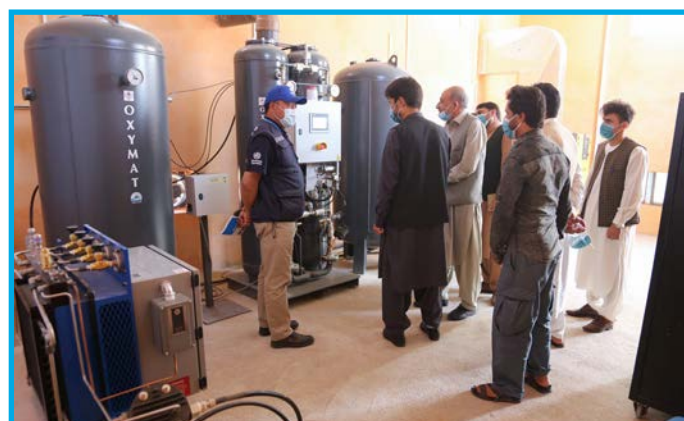
WHO inspecting oxygen processing at Herat COVID-19 Hospital.
