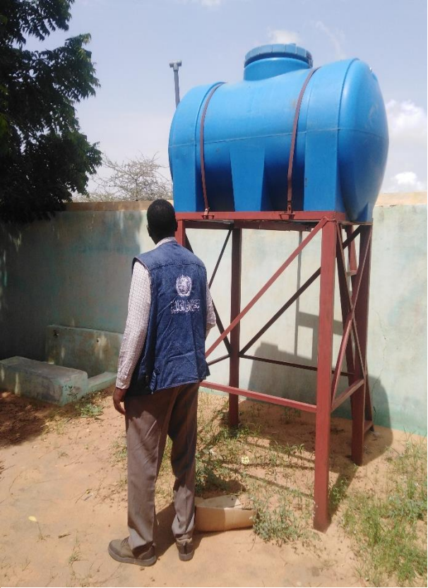
Figure 7: A water reservoir observed during the WASH assessment of one of the healthcare facilities in Sudan
