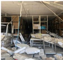
Heavily damaged central drug warehouse, WHO Lebanon
