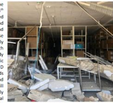
Heavily damaged central drug warehouse, WHO Lebanon
