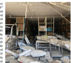
Heavily damaged central drug warehouse, WHO Lebanon
