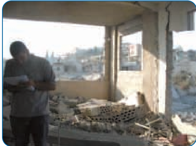
Filling the assessment questionnaire in one of the destroyed health facilities.
