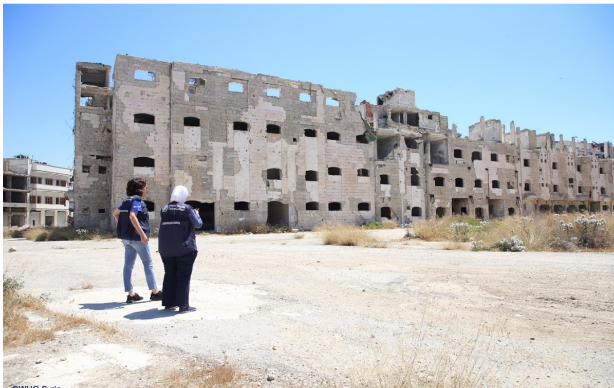
©WHO Syria Destroyed health facility in Homs governorate “Homs National Hospital”. The whole of Syria’s approach to the cholera response
